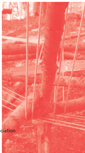
The Crossings Project A complex spaceframe of timber logs forms the structure of the bridge.
