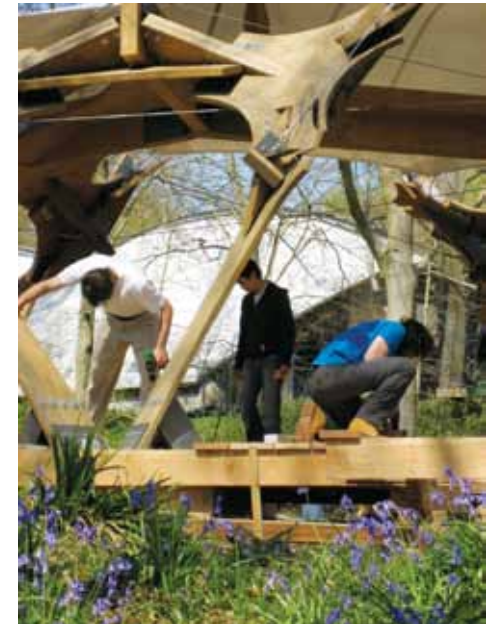
The 2006 AA Summer Pavilion, designed and built by Intermediate Unit 2, being re-erected at Hooke Park in 2007. Photo Martin Self
